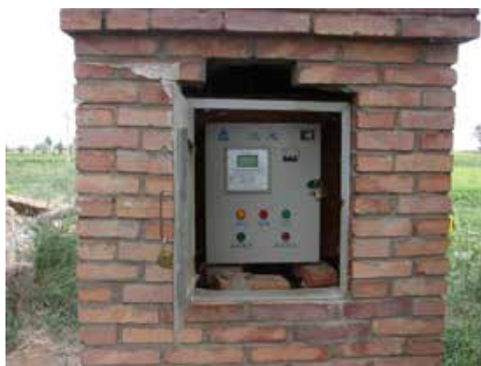
Smart card machine installed on pumping installation. Photo: Eefje Aarnoudse
